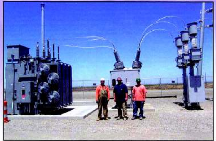
Alan Miller, James Bohacek, and James Kettlehake built the substation at the Contra Costa Water Pumping Plant.
