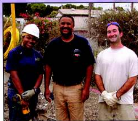
JATC Instructor and Del Monte Electric foreman Donald Dones (center) with apprentices Racheal Bryan and Ken Quigley at the Castro Valley library project.
