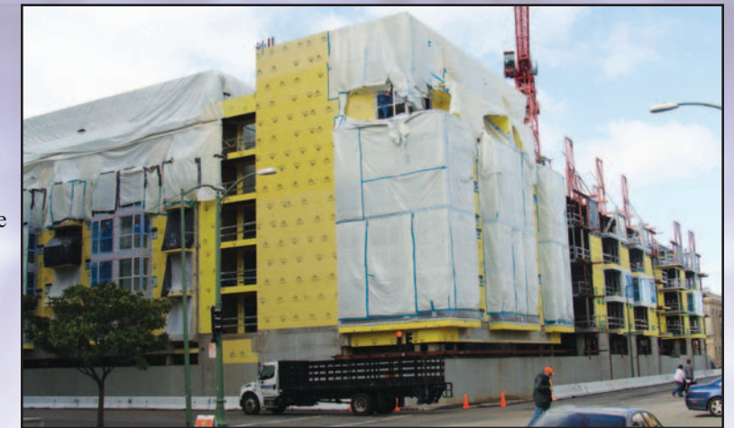
Blight in Oakland - The City Walk project, where non-union Helix Electric was working, has been sitting idle since July 2007. It is now being wrapped by its developer, the Olson Company, its future uncertain.
