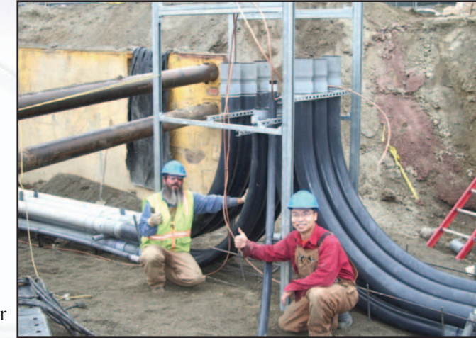
James Wray (left) and Kin Hui (right) finish installing 6" PVC coated rigid sweep elbows at the Mocho Groundwater Project in Pleasanton. Chris Senft, foreman for Blocka Electric, sent the photo with a big "thank you" for James and Kin.
