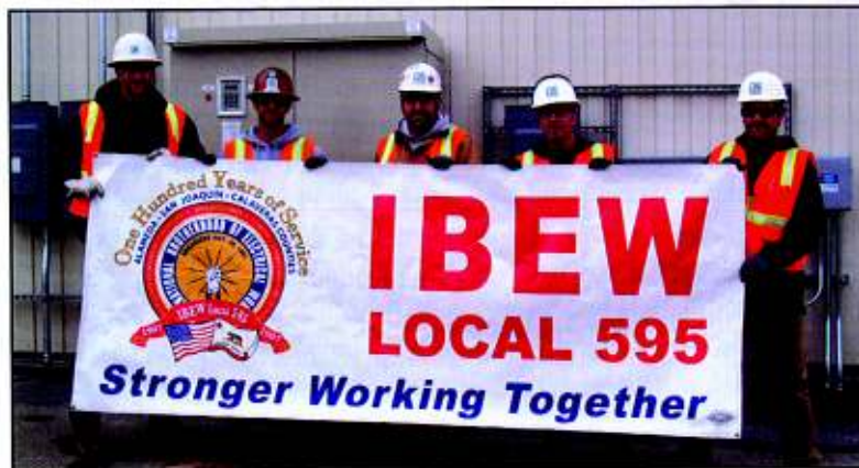
Vehid Husejnovic, Eric Harrison, Dave White, Brett Gibson and Steven Marchetti installing a PV system at Pleasanton's corporation yard.
